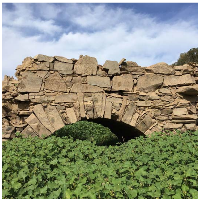
The North Fork Ditch from Auburn to Beals Bar was completed in late 1850s. In 1915 most of the ditch was lined in concrete to reduce water loss. This portion of the water canal is below Beals Point Park.
