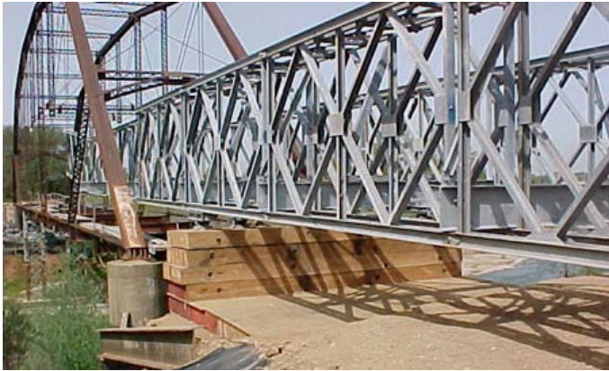
Preparing to remove the historic Meiss Road Bridge Photo: J. M. Turner Engineering Company
